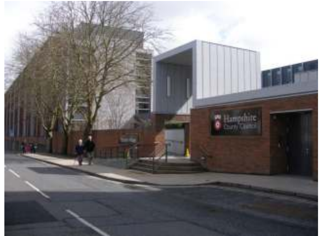
Fig. 5: Elizabeth II Court, Hampshire Council Offices, Winchester. The existing over 50yrs old concrete frame was retained, significantly reducing demolition waste, and the existing concrete cladding was removed, crushed and reused as aggregate in other materials. Previously hidden concrete soffits were exposed and painted, enabling the concrete, due to its thermal mass, to provide comfort and energy performance through passive design measures.
