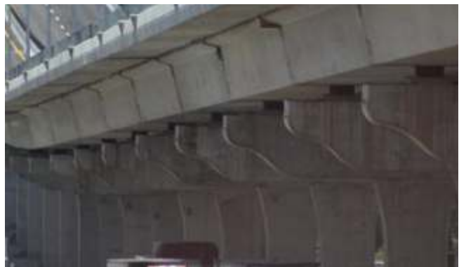
Fig. 14: Lead rubber base isolation bearings in the second floor of the Mexico-Puebla highway
