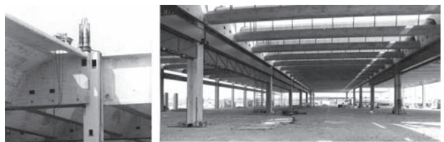
Figure 12. View of the connection at the top of the columns and of the factory bays
