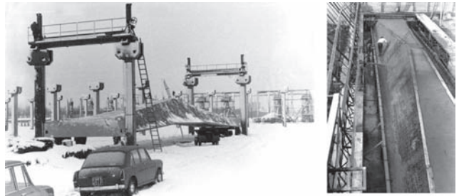
Figure 10. Views of the lifting equipment and of the use of the shotcrete
