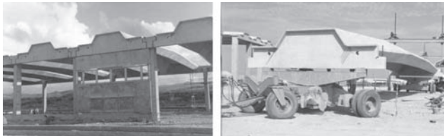
Figure 8. View of a factory under construction and of an unit being moved from the casting position
