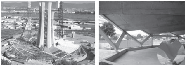
Figure 10. Scaffolding and forms for the shells and inside view of a lower one with the ball bearing detail
