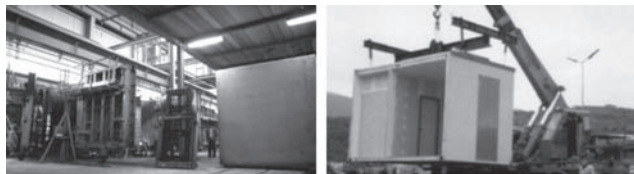
Figure 13. The form for the in the plan casting and the erection of an unit
