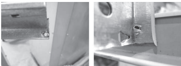
Figure 7. Failure mode in the rivet connection between the main beam and the wall angle
