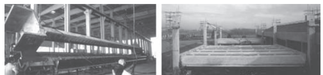
Figure 9. View of the demoulding and rotation of the shell and of the on site assembly of the roof unit
