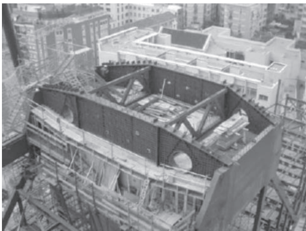
Fig. 8: Structural arrangement of the suspension head on top of the central core
