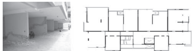
Figure 13: Building C, Viñadel Mar: general wall failure at first floor: 40 cm out of plumb at the top.
