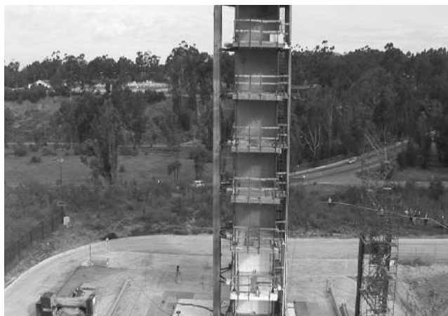
The Seven-Story Building on its Shake Table at the San Diego Super Computer Center, University of San Diego State (Courtesy: A. Chourasia)
