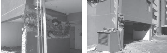
Figure 16: In building B; buckling of vertical reinforcement at wall discontinuity.
