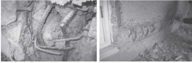
Figure 15: Buckling and fracture of vertical reinforcement at web and edge of an L shaped wall with opening
